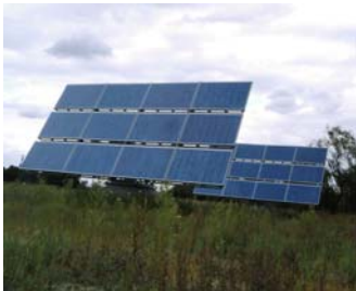
Photo-voltaic plant in Berlin-Adlershof Source: Wikipedia
